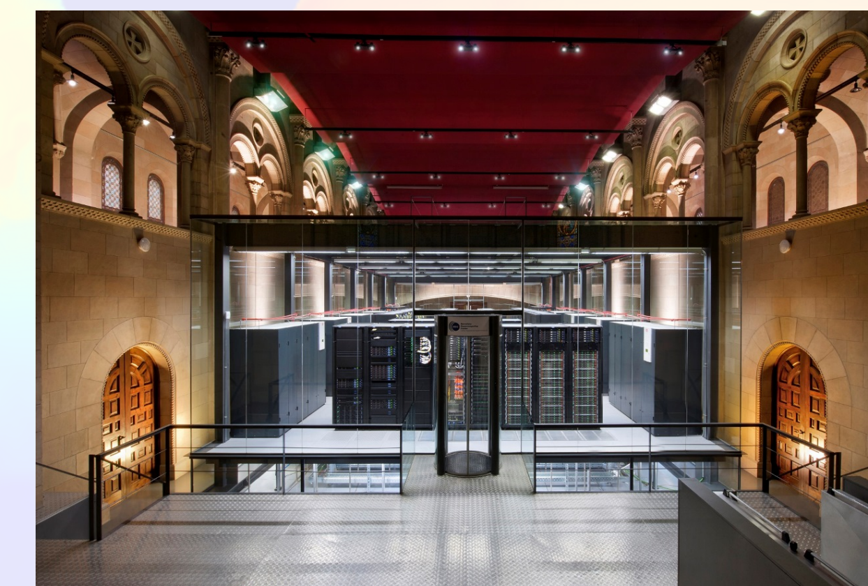
The MareNostrum supercomputer at the Barcelona Supercomputing Center
